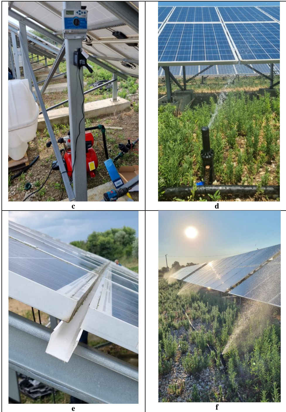
Fig 6. Components of the cleaning system and pre-trails.
