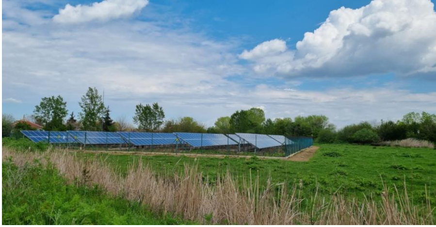
Fig 5. Solar power plant
