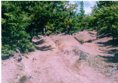
Fig. 11: The rural road in the river basin damaged by water induced erosion.
